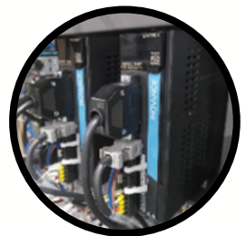
Gantry is controlled by metal encoder and 750w AC motors
